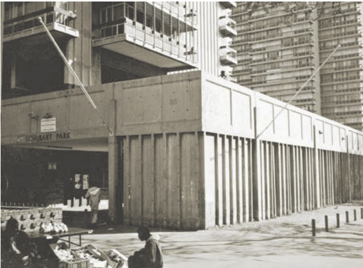
The dilapidated Schubart Park flats in Pretoria – a well-known landmark in central Pretoria and a typical example of urban decay.
